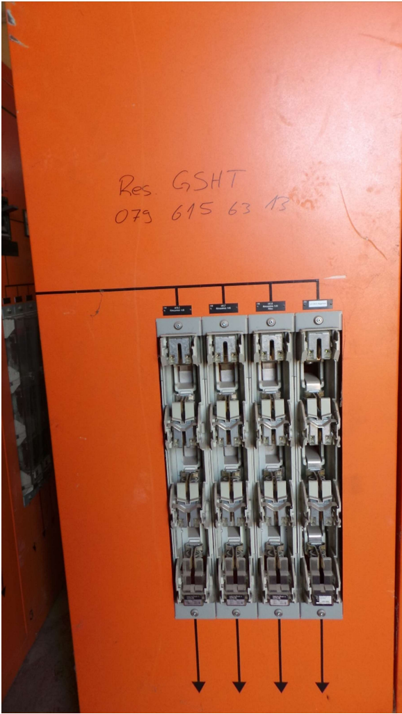
Part of low tension Distribution
